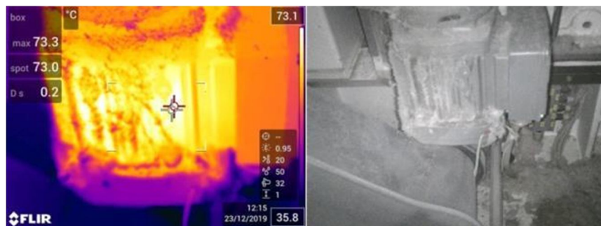
Figure 7. Card feed motor at card no found heated condition a) IR Image b) Visible Image
