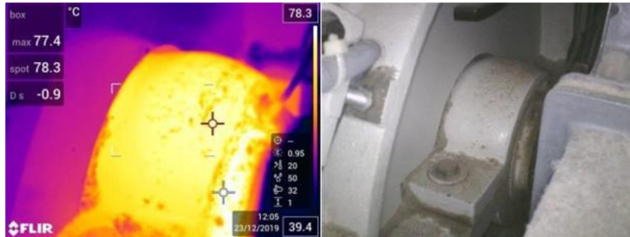
Figure 6. Cylinder bearing housing at card no-3 found heated condition a) IR Image b) Visible Image
