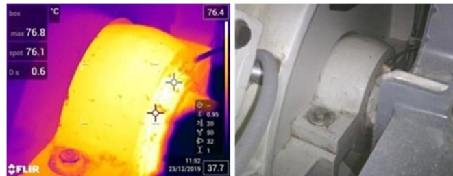
Figure 3.4. Cylinder bearing housing lhs at card no-1 found heated condition a) IR Image b) Visible Image
