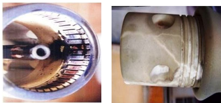
Figure 2. Sample photos of deteriorated contact
