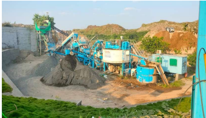
Figure No 1: PCMC C&D Waste Recycling Plant
