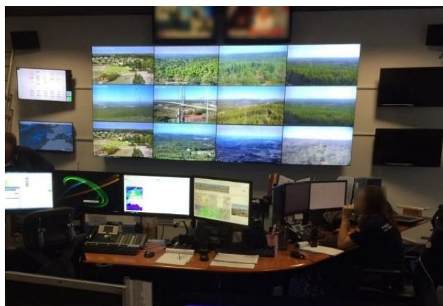
Figure 4. Command and control center with video wall
