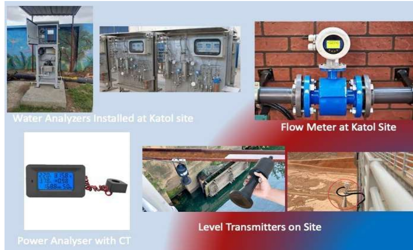
Figure 1: Inline sensor installation at WTP
