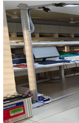
Figure.10 Solar Powered Smart Lamp Post
