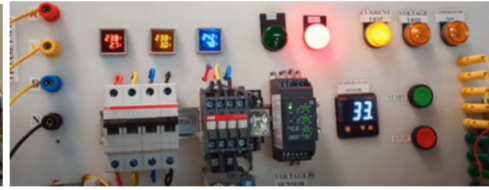
Fig 14: Kit after overcurrent fault occurs
