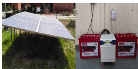
Fig. 5: A solar photovoltaic system with a power control unit designed for cold storage
