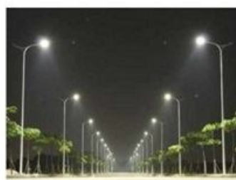
Figure 2.4 Sensor Installed in Lamp Post, Kolkata
