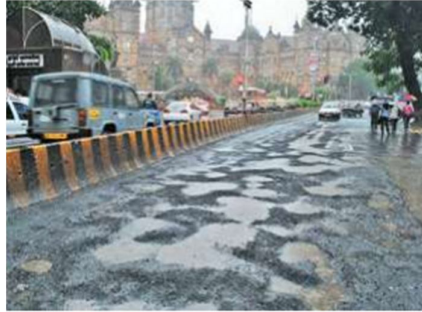
Figure 1. Potholes on the road
