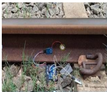
Figure 1. A railway track's location of a vibration sensor
